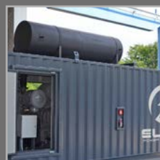
Residential Muffler on the roof it guarantees an acoustic reduction of the exhaust noise
