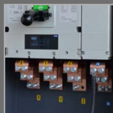
Connection copper bars where provided they allow to connect more cables on the same phase
