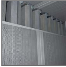
Air intake louvres and special attenuators prevent noise dissipation
