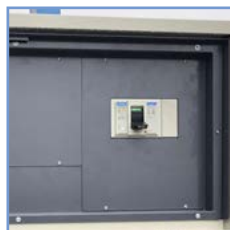
General switch mounted on the panel for a comfortable and safe connection
