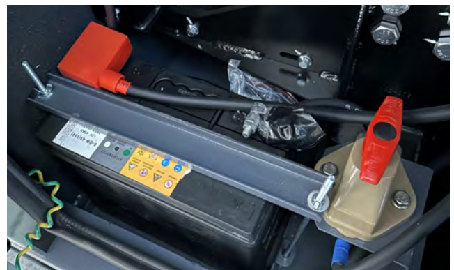
Battery isolator for maintenance and storage
