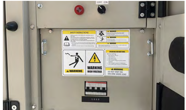
Panel with door, keylock and porthole
