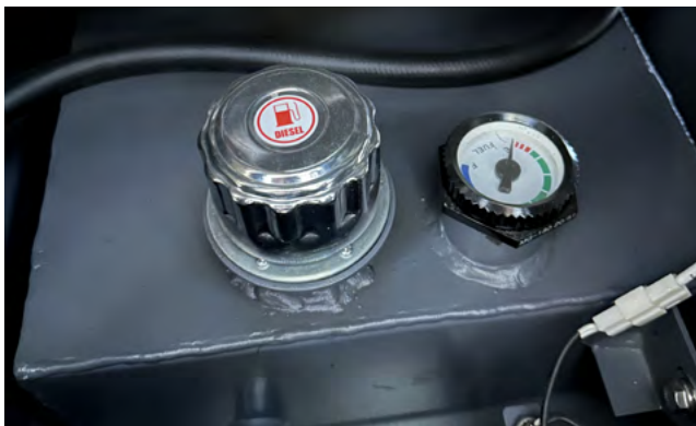
Tank with wide tank refilling point and fuel level indicator
